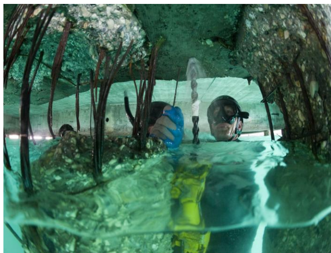
(Before Repair) 80% of all support piles were damaged this badly or worse
