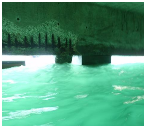
(After Repairs) Forms were placed around each pile and concrete was poured
